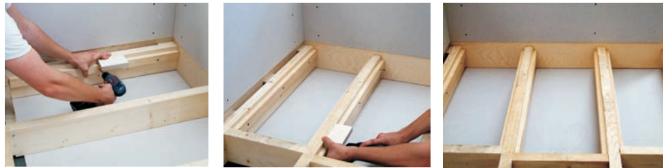
6. With an off cut from the waste support as a guide secure 50mm x 25mm softwood battens 24mm below the top of the joists to both sides of the joists over the area of the tray using 50mm X No 8 countersunk wood screws @ 150mm centres.
