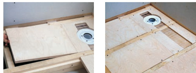
10. Cut and lay pieces of 24mm plywood between the joists to form a false floor. Secure the plywood and waste support to the joists and battens using 50mm X No 8 countersunk woodscrews @ 225mm centres.
