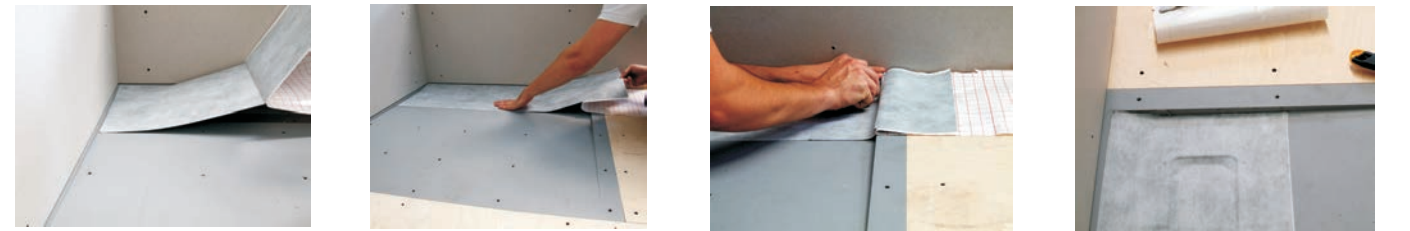
15. Lift up the tanking mat and gently removing the backing tape approx 300mm at a time, apply pressure to the mat and stick down. Fold the mat into the tray the other end and trim with a sharp knife.
